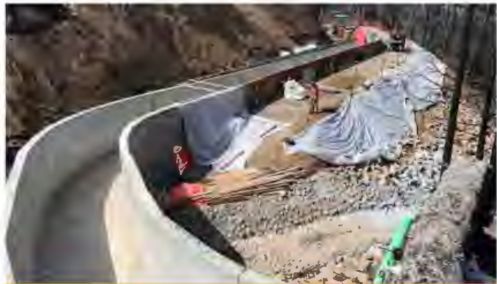
The Caldor Wildfire burned through EID’s Flume 4, 5, 6, and 30 in August 2021. Reconstruction of these flumes began in September 2021 and are now complete.
