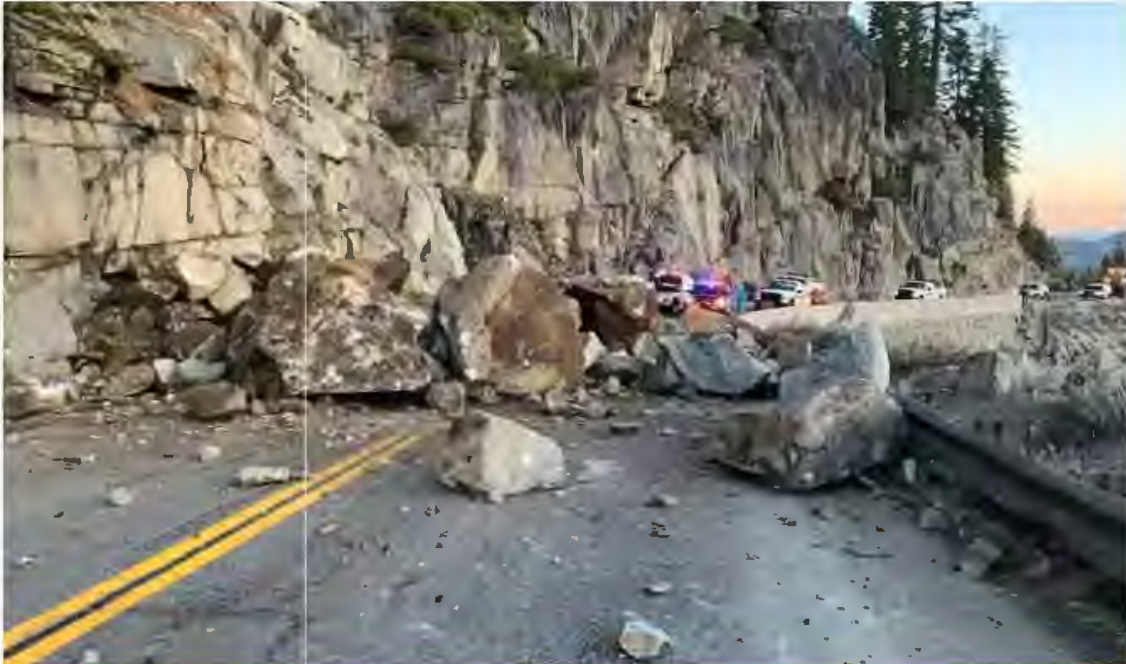
State Highway 50 along Echo Pass closed in April 2019 after a rockslide occurred and caused a collision.
