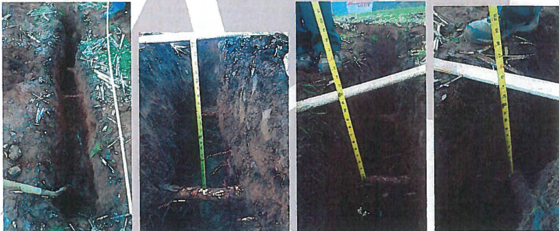
Ten foot long, two-foot deep trench excavated 16 feet from trunk. Two roots were observed. The impact to tree from root pruning of these two roots at this point from the trunk is considered low.
