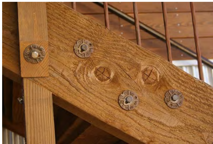
Visible Fastenings in Wood Elements at Diamond Center
