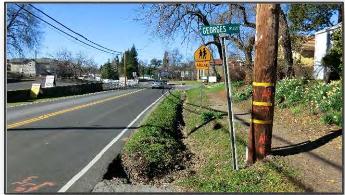
Worn pedestrian path on Pleasant Valley Road
